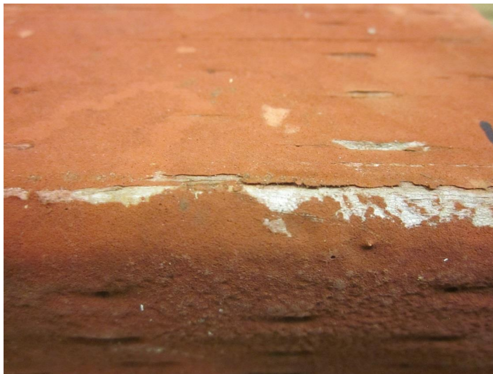
Figure III-4. Photos of the upper surfaces of coated, non-treated control samples after 6 years of exposure in Hilo, Hawaii showing erosion of the coating and complete loss of coating on the corner.
