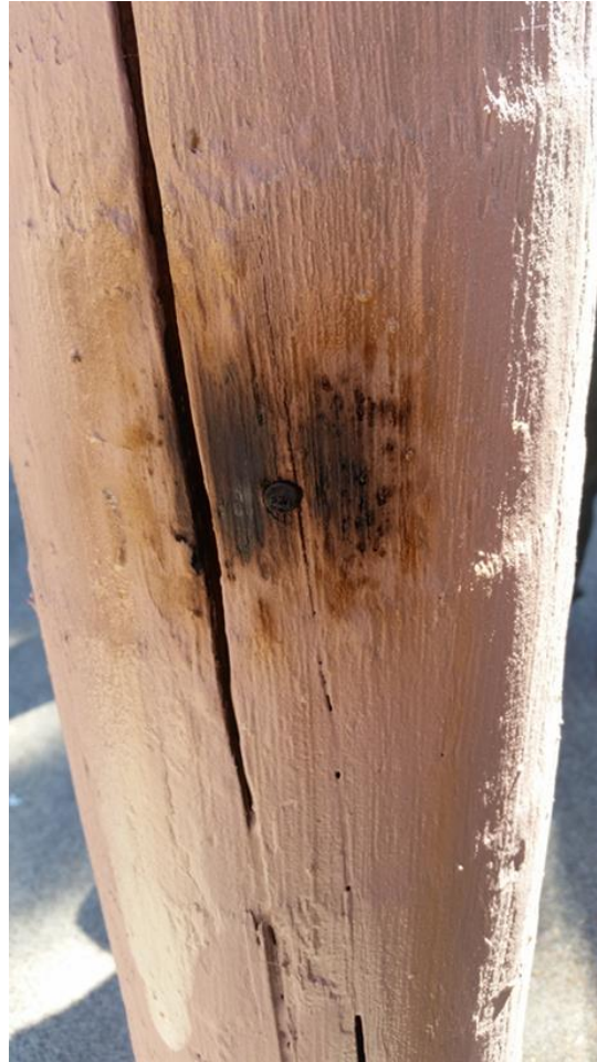
Figure III-17. Example of a FireGuard treated pole section showing slight charring where the barrier was sacrificed.
