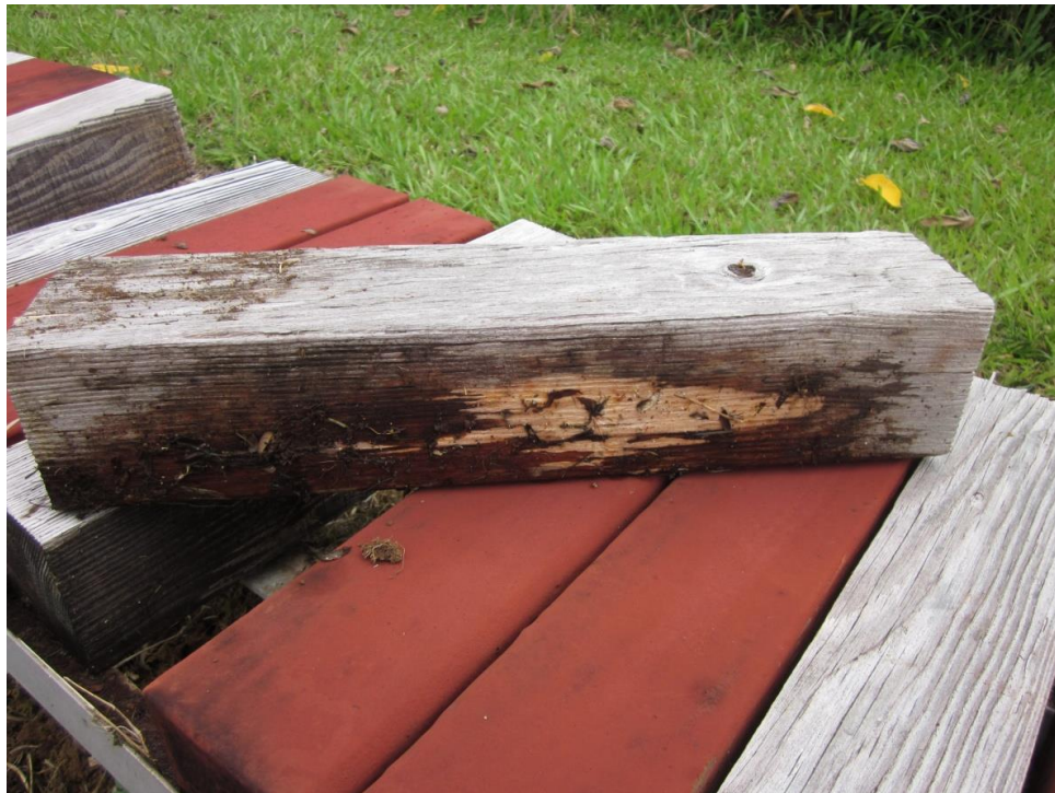
Figure III-3. Example of a non-treated, non-coated wood sample after 6 years of exposure in Hilo, Hawaii showing evidence of fungal decay and fruiting bodies.
