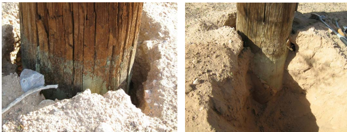
Figure IV-1. Poles in the APS system after excavation showing evidence of animal gnawing on the barrier bandage.
