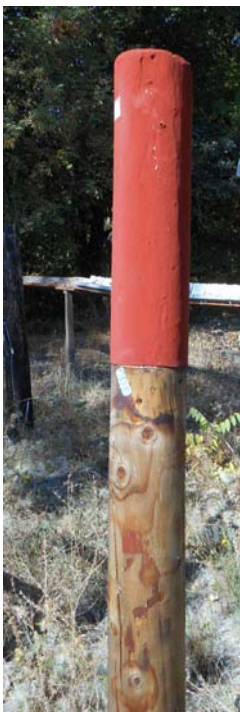
Figure III-35. Example of a polyurea coated pole top.
