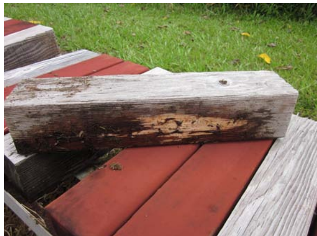
Figure III-14. Example of a non-treated Douglas-fir crossarm section with visible decay after 4 years of exposure in Hilo, Hawaii.
