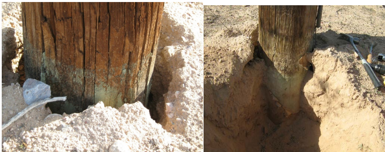
Figure IV-1. Poles in the APS system after excavation showing evidence of animal gnawing on the barrier bandage.
