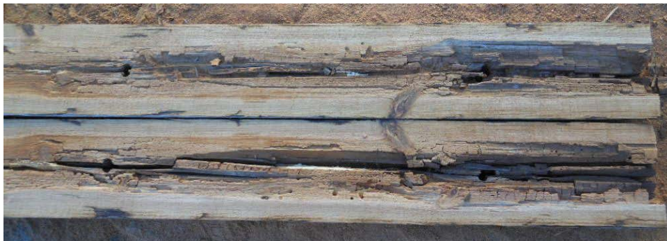
Figure III-30. Longitudinal section through a pole showing a woodpecker gallery associated with extensive internal decay.
