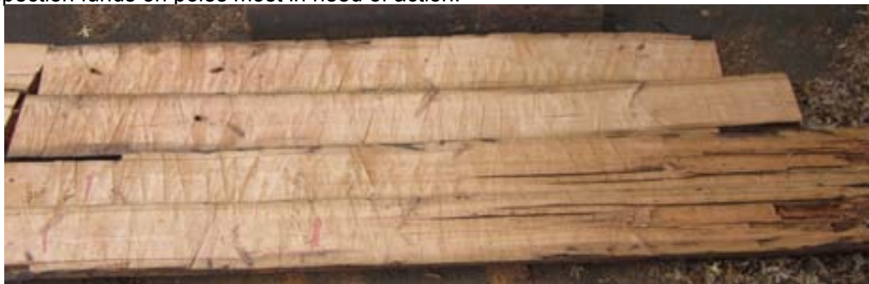
Figure III-27. Longitudinal cross section through a two part of a pole showing clear wood near the butt (top section) and extensive internal decay near the top (bottom section).
