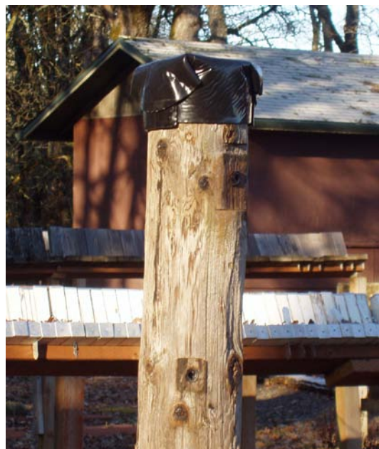
Figure III-33. Example of a capped pole used to assess the effects of capping on wood moisture content.
