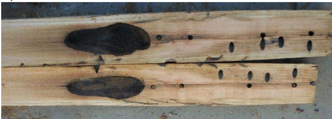
Figure III-31. Longitudinal section through a pole showing a wood pecker entry point and some associated damage. This pole corresponds to the images in Figure III-c.
