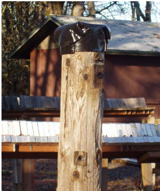
Figure III-7. Example of a capped pole used to assess the effects of capping on wood moisture content.
