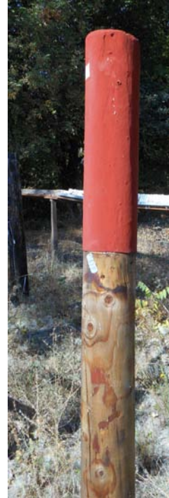
Figure III-9. Example of a polyurea coated pole top.
