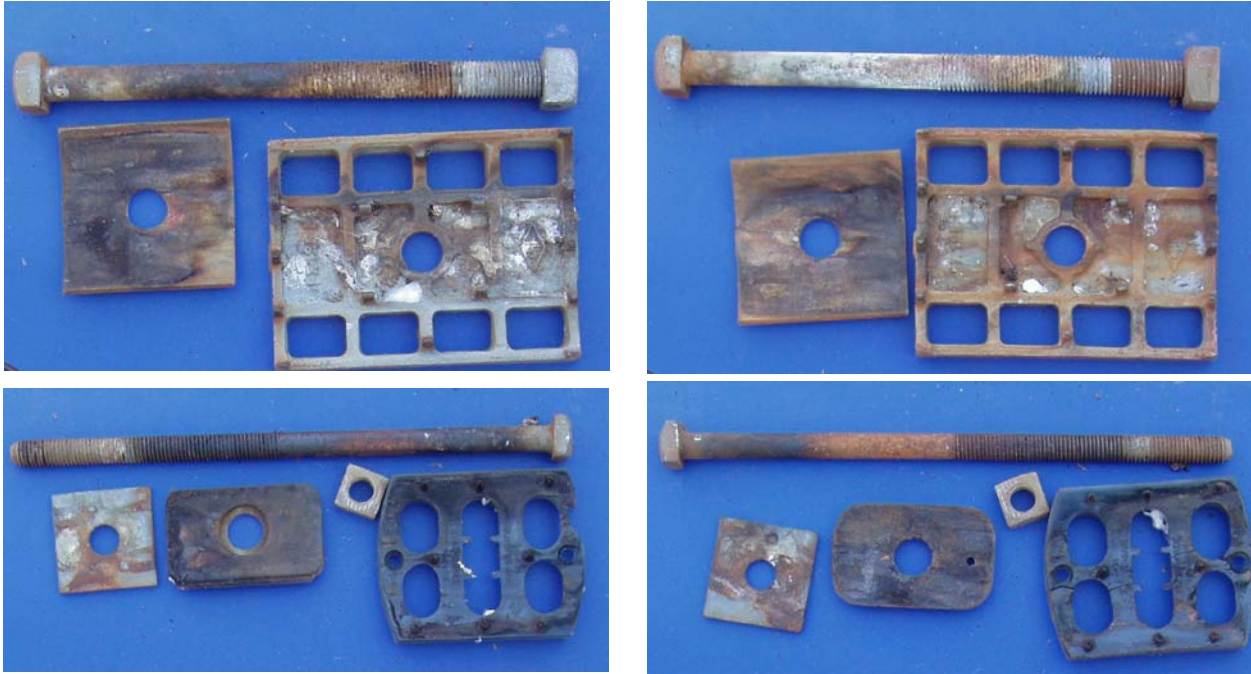
Figure II-2. Condition of nuts, bolts and gain plates removed from field drilled bolt holes 32 years after treatment of the exposed non-treated wood with boron (Polybor) prior to bolt insertion.
