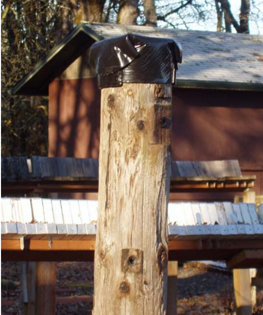
Figure III-8. Example of a capped pole (Osmose Pole Topper) used to assess the effects of capping on wood moisture content.
