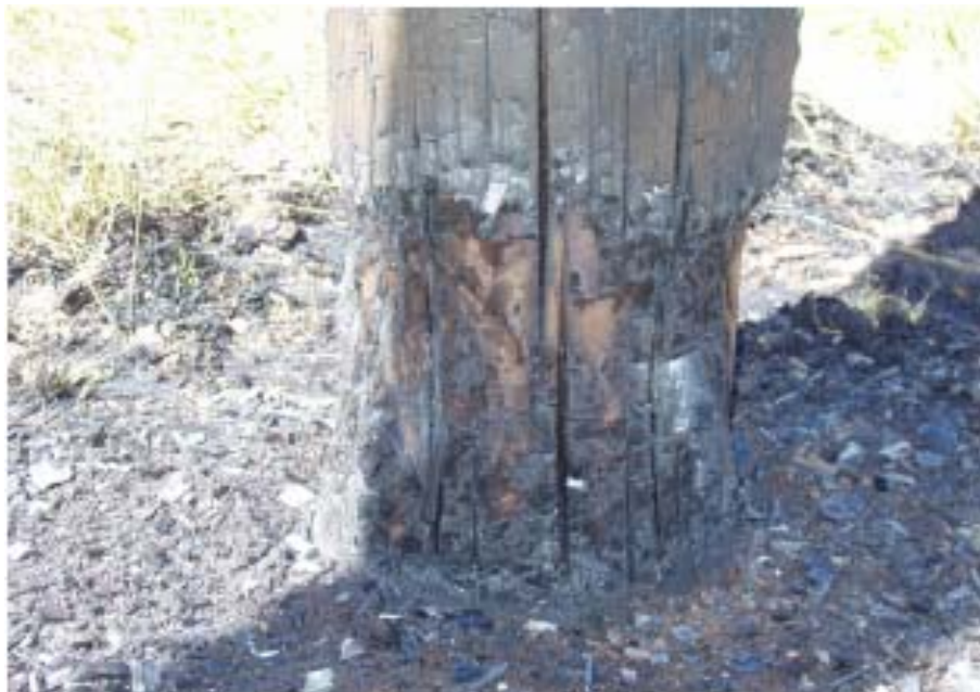
Figure III-7. Example of char around a pole following a fire test.
