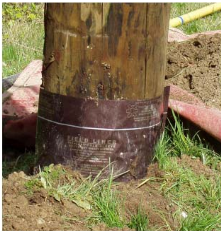
Figure III-5. Example of external barrier assessed on Douglas-fir poles.
