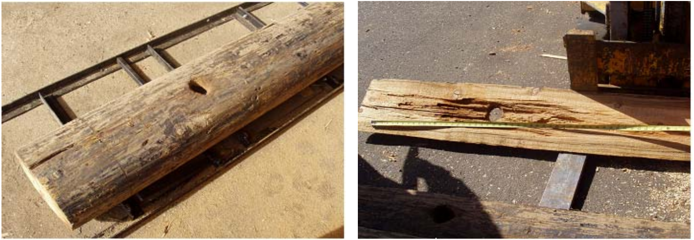
Figure III-12. Example of sections through a Douglas-fir pole showing a woodpecker hole on the surface and the extent of the internal damage associated with the hole.
