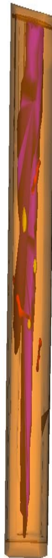
Figure III-14. Illustration of reconstructed internal damage in a Douglas-fir utility pole after 25 years in service.
