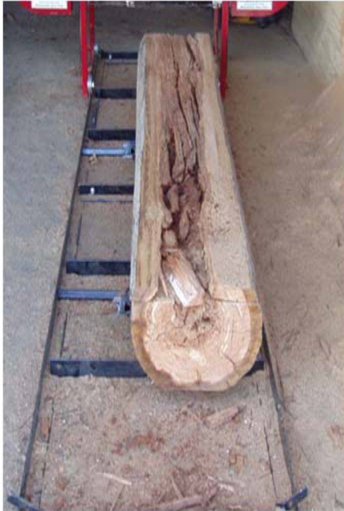
Figure III-11. Example of a section through a Douglas-fir pole showing internal decay.
