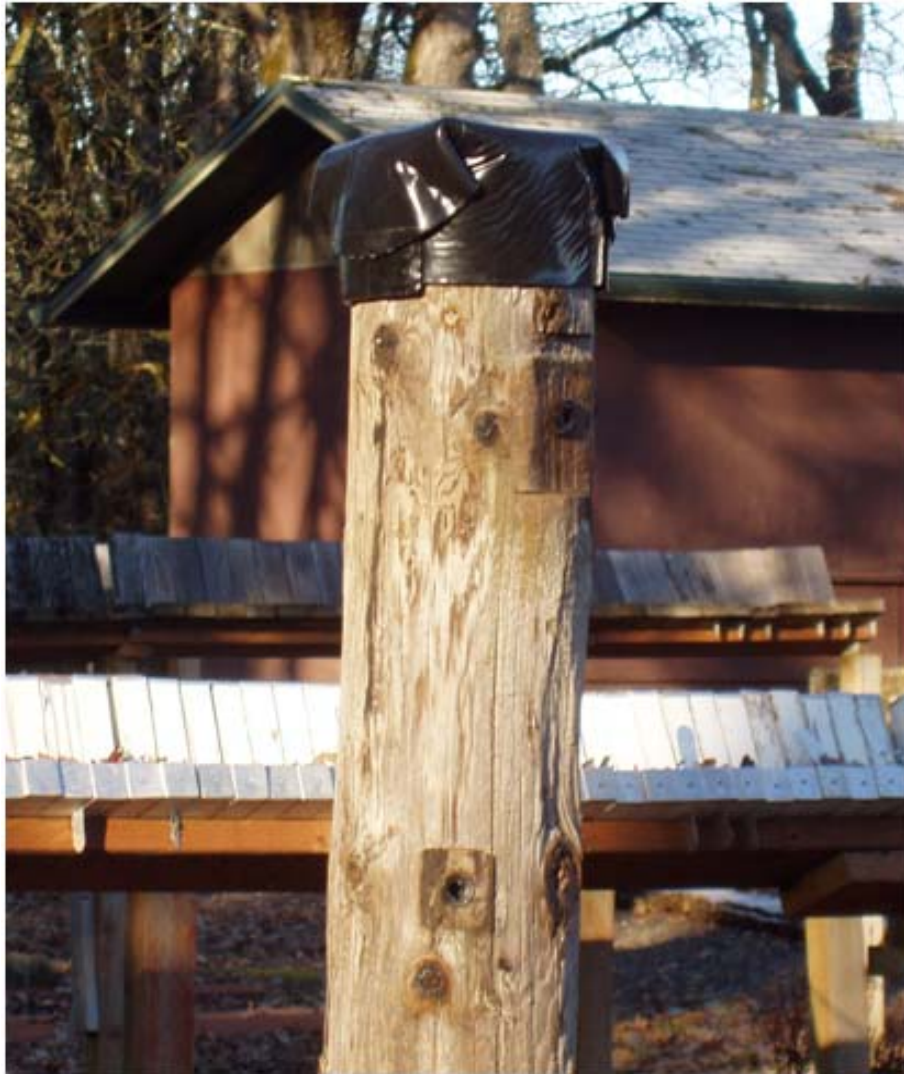
Figure III-15. Example of a capped pole used to assess the effects of capping on wood moisture content.
