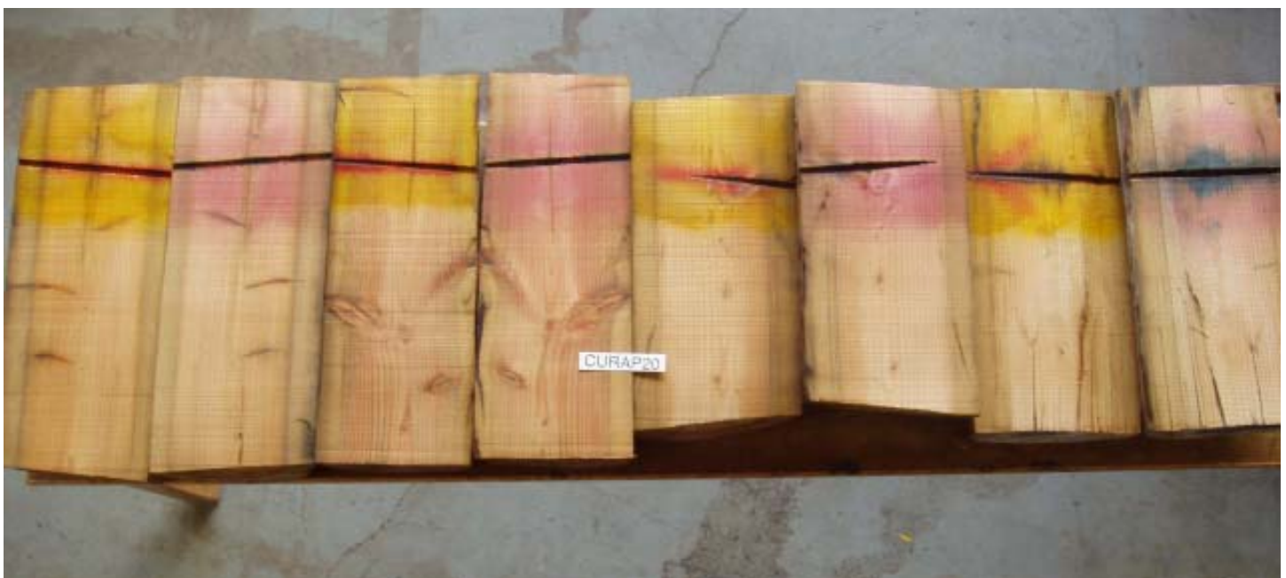
Figure II-4. Degree of copper and boron movement away from the sites in Douglas-fir pole stubs where CuRap 20 coated galvanized threaded rods were installed six years earlier. Red indicates the presence of boron and blue-green indicates the presence of copper.
