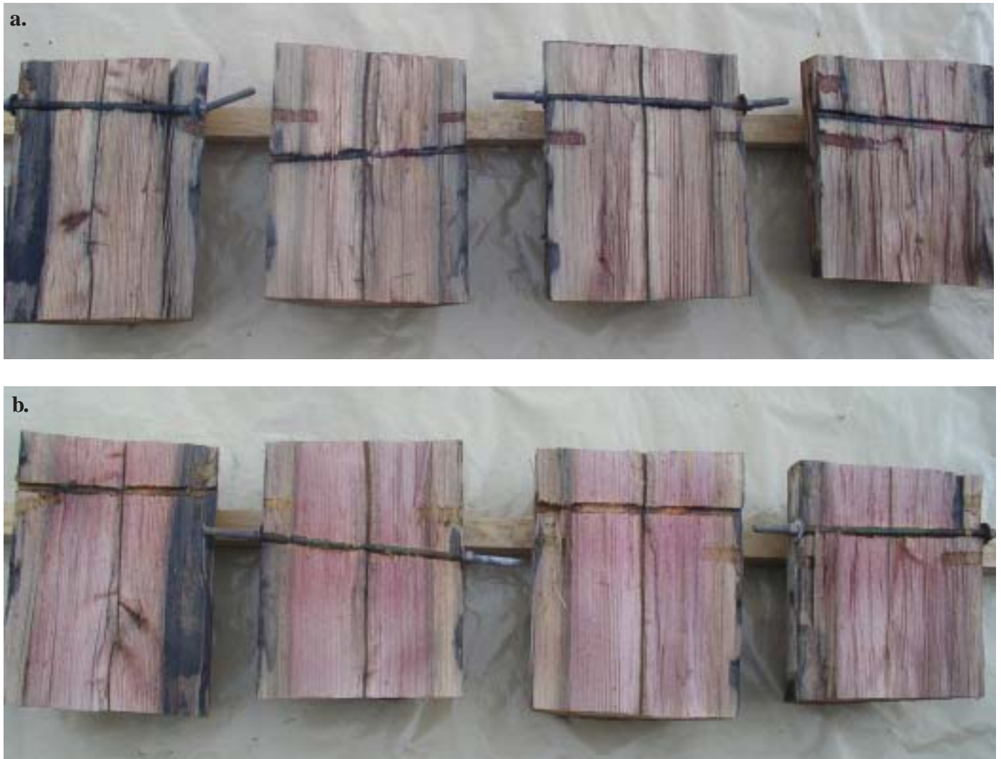
Figure II-2 Degree of a) copper [blue color] and b) fluoride [yellow color] movement away from the sites in Douglas-fir poles where Cop-R-Plastic coated galvanized rods were installed three years earlier.
