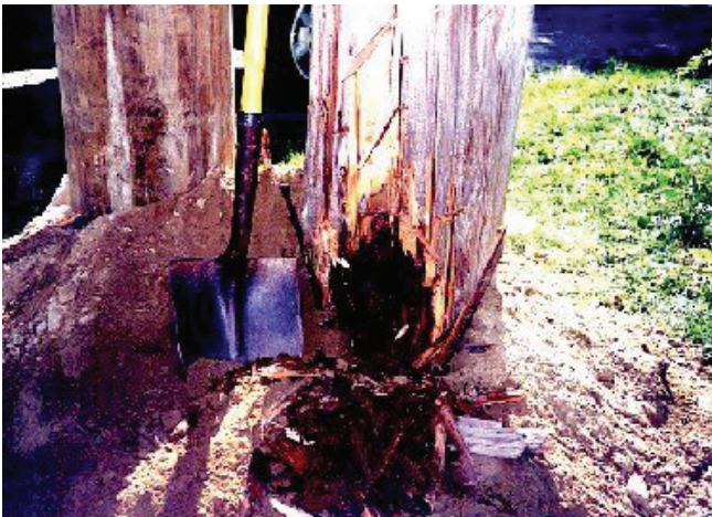
Figure 22. Carpenter ant damage in poles. Carpenter ants also live in colonies, hollowing out nests in poles for shelter. A pile of sawdust at the base of the pole is a sure sign of their presence.
