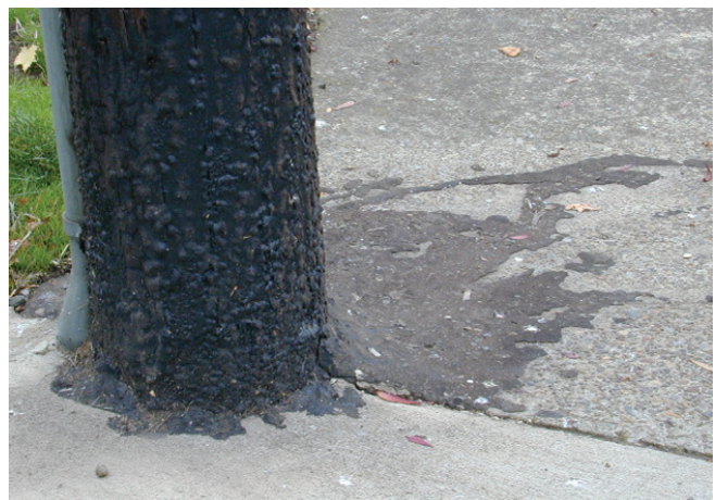
Figure 11. Example of bleeding from a creosote-treated pole.
