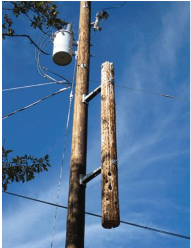
Figure 25. A section of old pole containing a woodpecker nest attached to a new pole in hopes of discouraging new attack.
