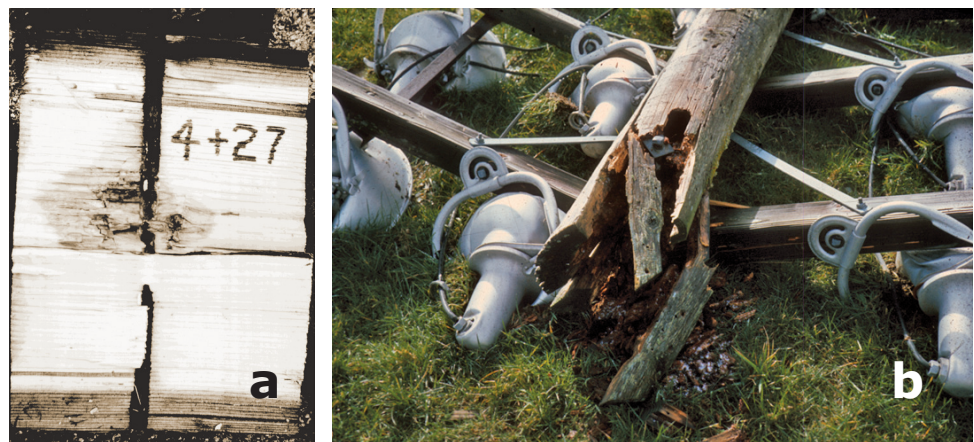
Figure 4. (a) Decay at the bolt hole and (b) pole failure caused by decay in a field-drilled hole.
