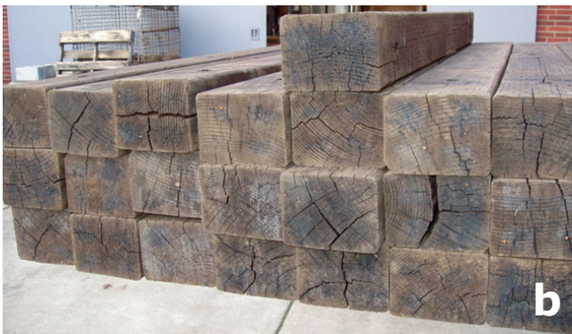
Figure 27. Crossarms (a) with and (b) without end-plates that limit end-checking. Note the large checks on non-plated ends.
