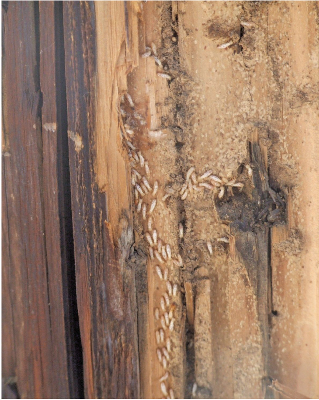
Figure 20. Example of termite damage to wood. Note the debris and termite excrement on the wood.
