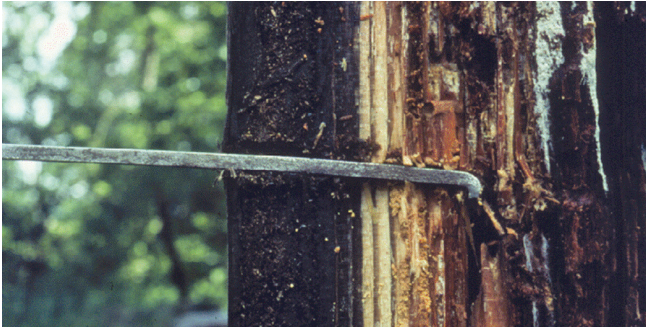
Figure 36. A shell-thickness indicator detects rot in poles by "feeling" growth rings in sound, but not rotten, wood when inserted or removed from snug-fitting holes.
