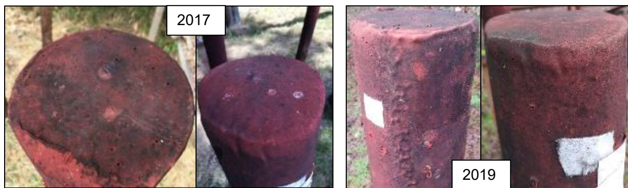
Figure 3.1.3. Condition of polyurea coatings on the tops of Douglas-fir pole sections after 73 months (left) and 90 months (right) of exposure in Corvallis, OR.
