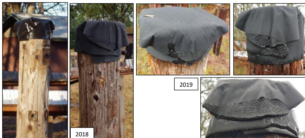
Figure 3.1.1. Example of the condition of water-shedding caps at the start of exposure and after 126 and 142 months of exposure in Corvallis, OR.
